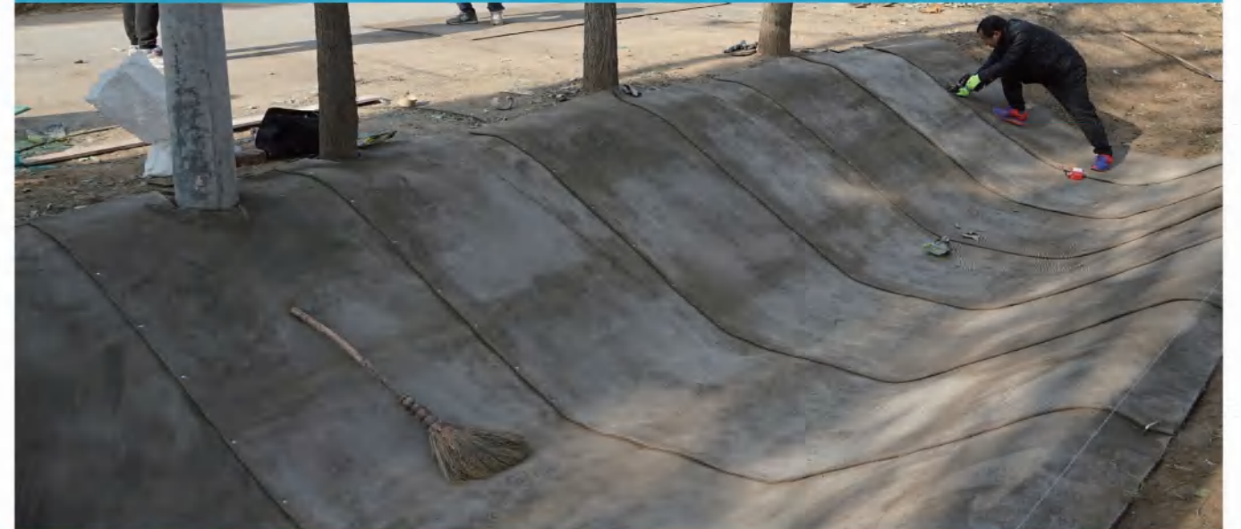
Oil storage area protection
